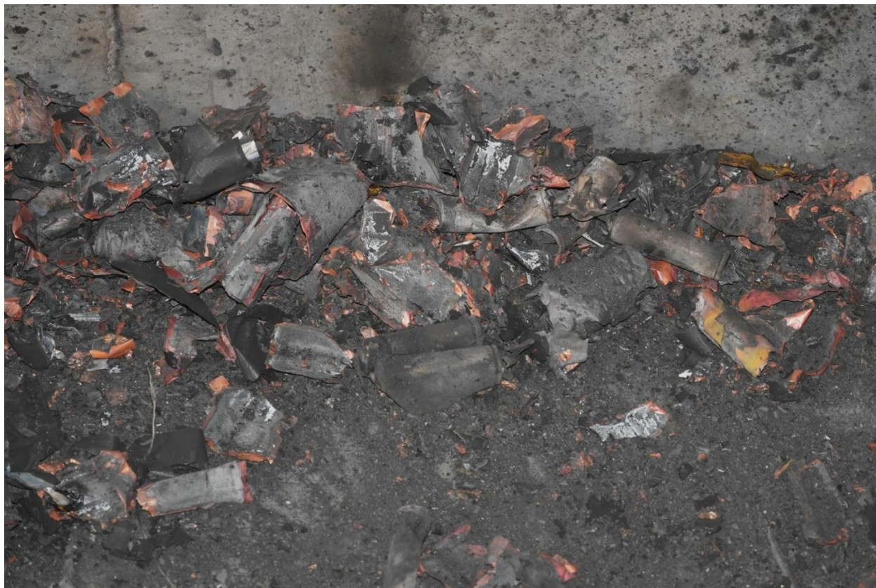
Figure 107. Close-up of the debris from the inside of the battery.
