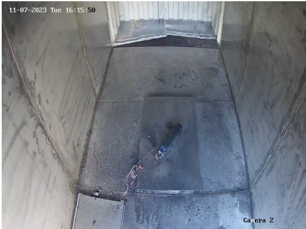
Figure 57. No visible smoke from battery.
