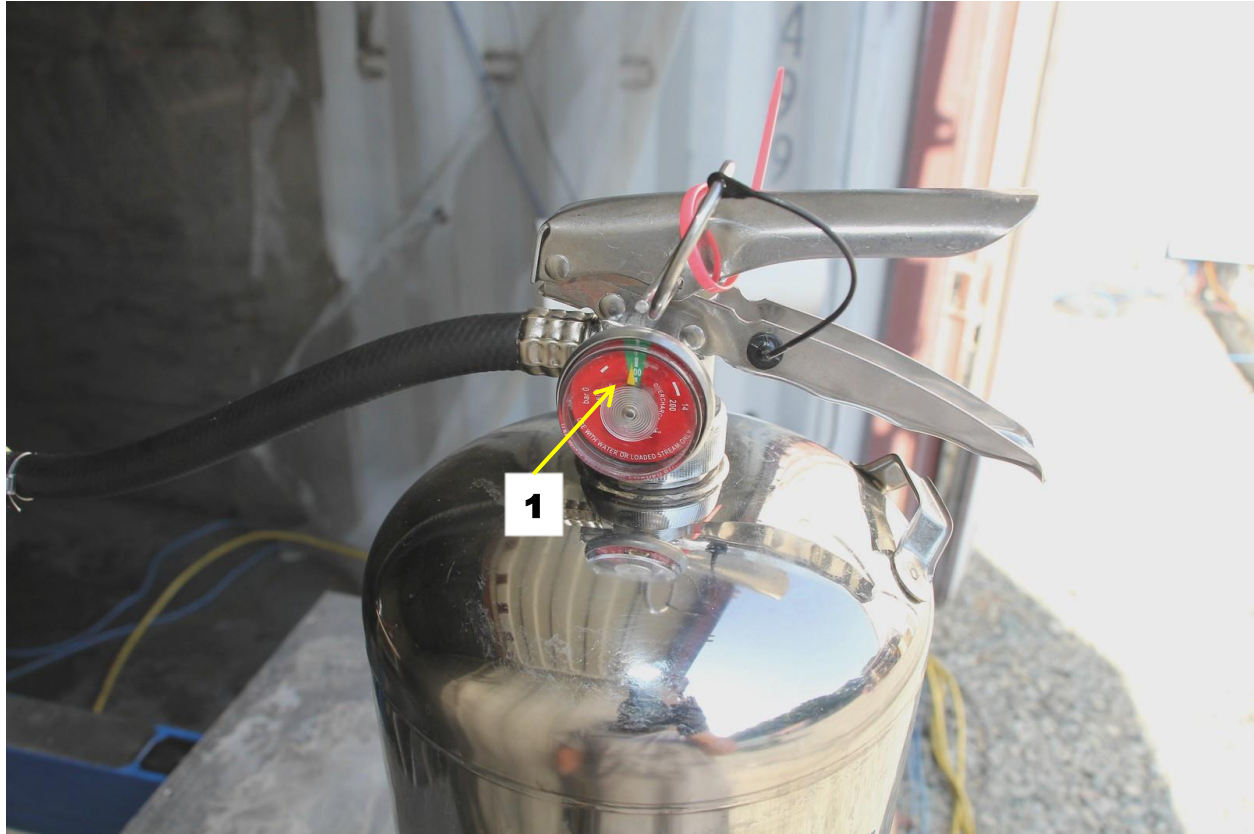
Figure 7. Charged fire suppression canister.
