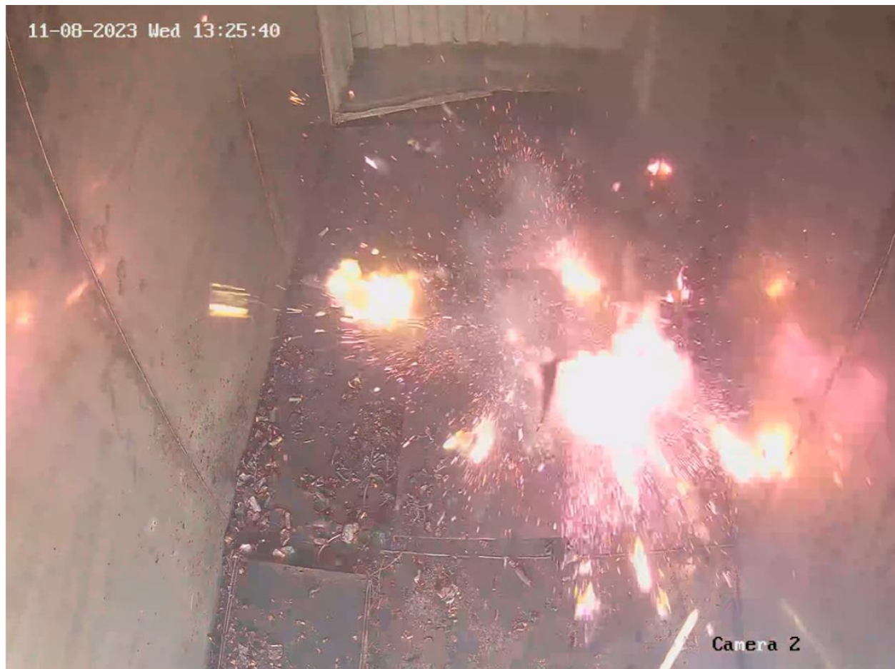
Figure 102. Final cells going into thermal runaway.
